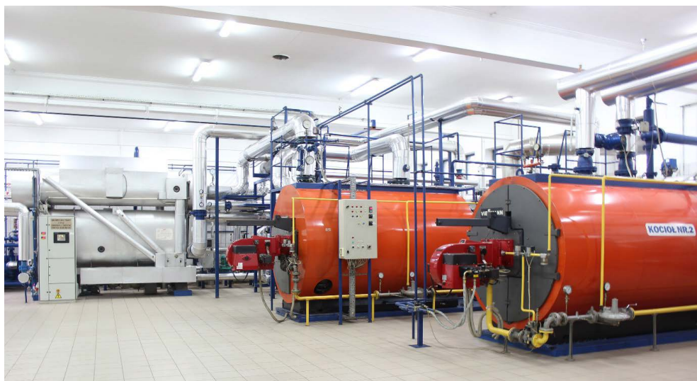
Fig. 42. Gas boilers in the Geothermal Heating Plant in Mszczonów (photo: M. Słowek)
