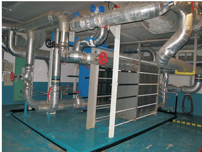
Fig. 6. Titanium heat exchangers of a geothermal installation with Dogger water
